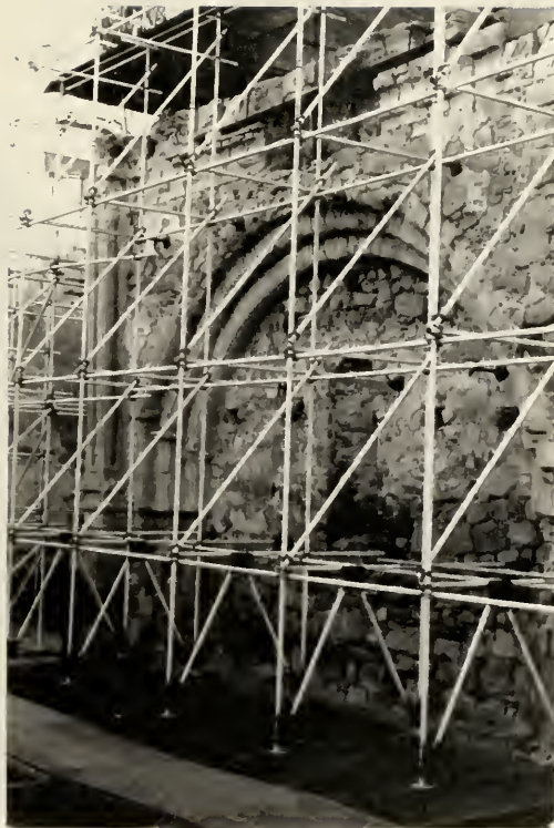
Fig. 4. View of east wall of nave, Old Stone Church (1994). The load-bearing stones are green and yellow sandstone. The stones in the cornice and pilaster are volcanic tuff, and the stones in the arch yellow sandstone and tuff. Fragments of lime-based plaster are present below the cornice and arch.
